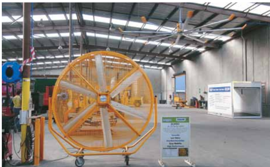
Tieman has installed an 8m span Big Ass fan into the workshop ceiling. Also pictured is a mobile AirGo Big Ass fan.
