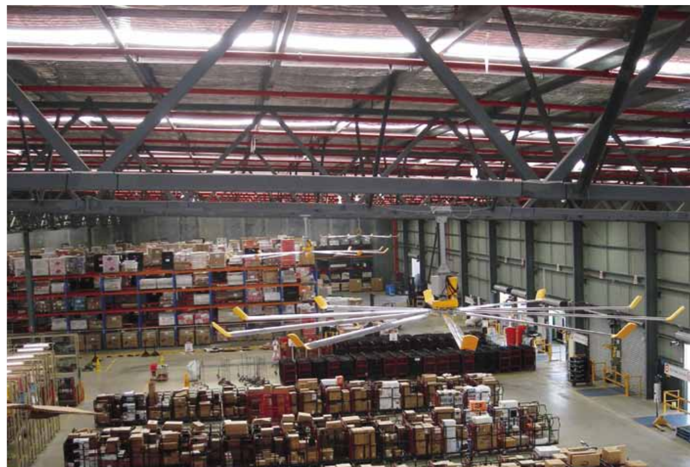
A series of Powerfoil fans shown along the length of warehouse.
