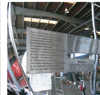
All signage is stainless steel with additional operational valve matrix sign.
