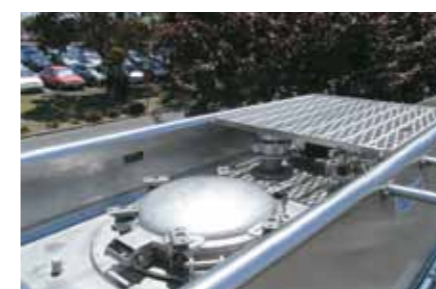
Hinged mesh platform for standing when in gantry area.
